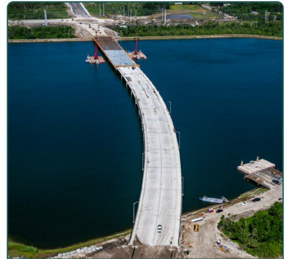
Looking west over the new bridge across South Lake leading into the new Lena Road Roundabout and the I-75 Overpass bridge
