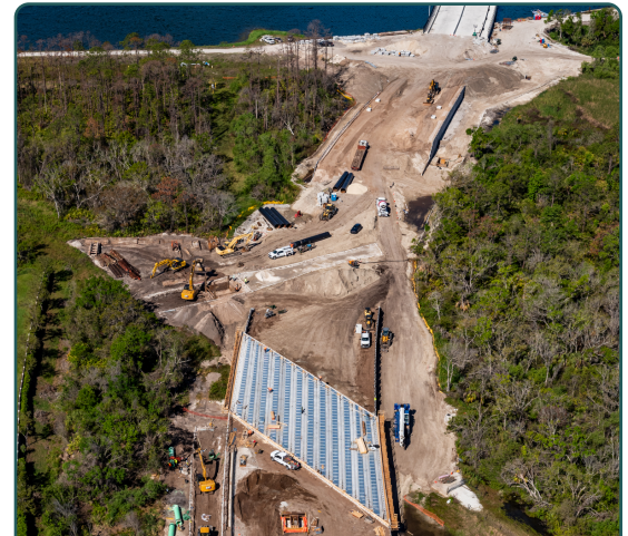
Bridge deck formwork and other construction activities progressing east of the South Lake bridge in preparation for the 44th Avenue East extension to Lakewood Ranch Boulevard.
