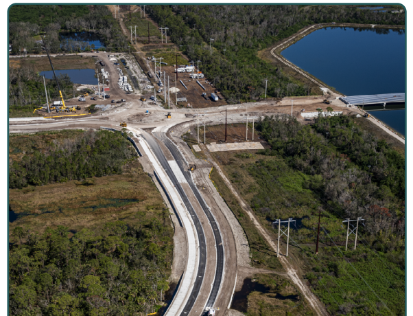
Northward-facing view of construction east of I-75: Northern extension of south Lena Road to the new 44th Avenue East roundabout
