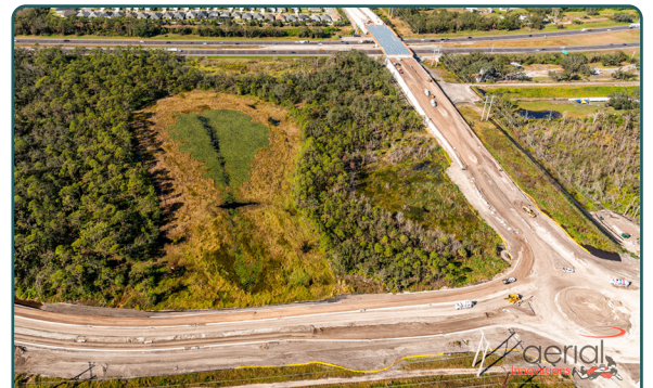
Construction at the eastern end of the bridge over I-75, and the new 44th Avenue East roundabout and connection to south Lena Road
