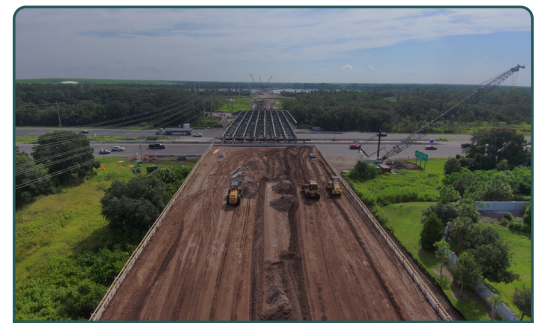
Roadway construction activities on the 44th Avenue East bridge approach west of I-75
