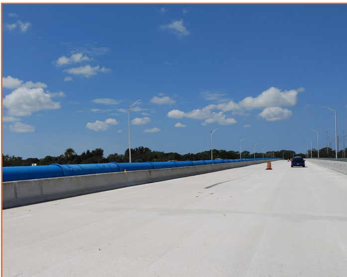
A westward view traveling on the 44th Avenue Bridge over the Braden River
